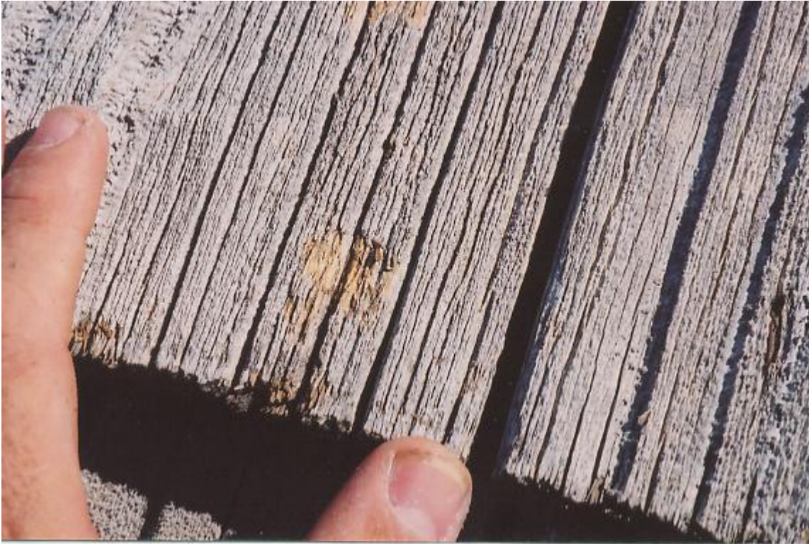
Age related cracks do not qualify as hail damage.
