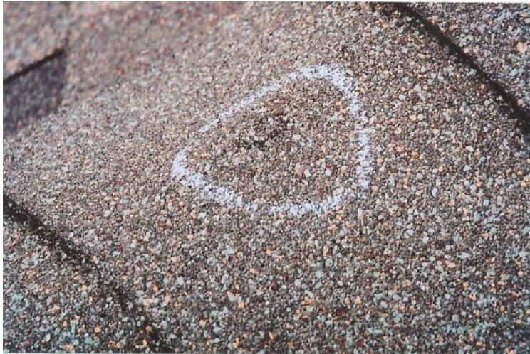
Hail often damages ridge shingles.
