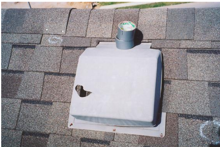
Hail hits can leave large leak-prone holes in vents. Duct tape can provide a quick emergency repair.
